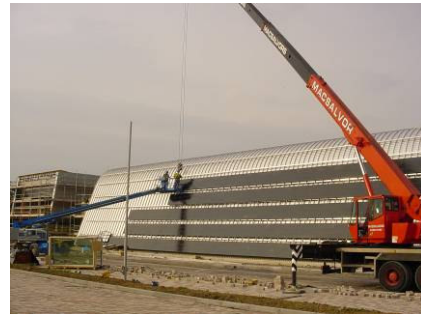
LSBIPV – OpTIC Centre, Wales
