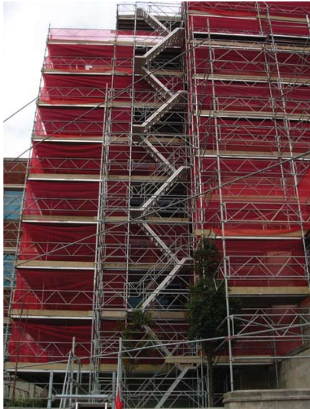
Figure 4 Stair towers provide good access. Make sure they are properly secured and erected (Image courtesy of Turner Access)
