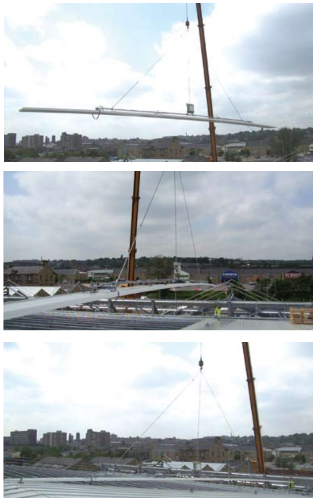
Figure 41 24 m long roof panels being mechanically lifted from ground level and installed on roof (a) (b) (c)
