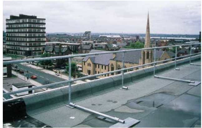
Figure 45 Permanent guard rail retrofitted during refurbishment work. Similar protection can be included in initial designs
