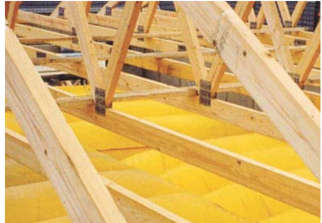
Figure 15(b) Air bags being used as a fall mitigation measure during roof work (Image courtesy of Airtek Safety Products Ltd)
