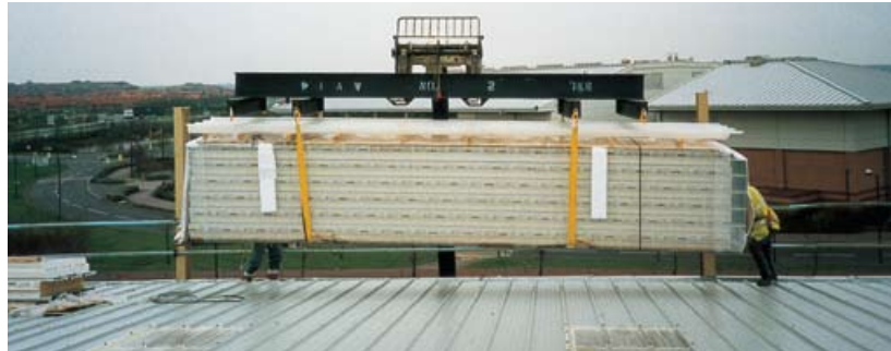
Figure 34 Delivering sheets to roof level onto the completed load-bearing section and behind the leading edge. (Note that the roof lights include mesh protection and are non-fragile)
