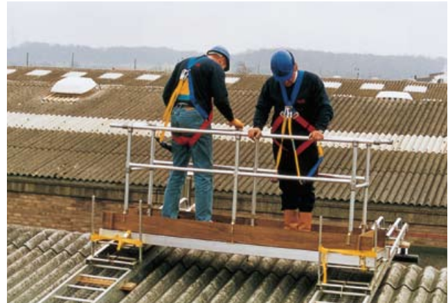
Figure 14 Access system for short-term maintenance work on a fragile roof
