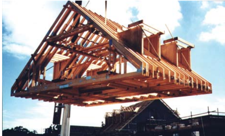
Figure 22 Craning a pre-assembled roof into position greatly reduces the need for work at height (Image courtesy of the Trussed Rafter Association)
