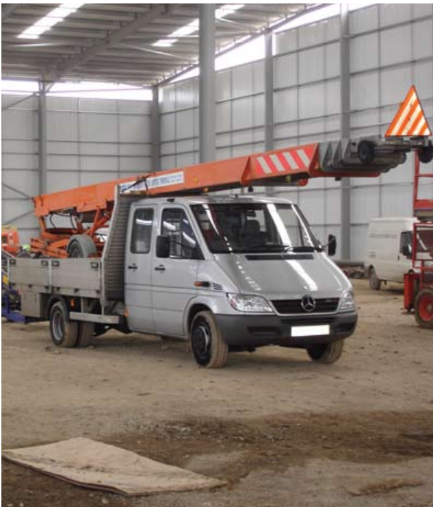
Figure 40(a) Mechanical handling of large roof sheets (Images courtesy of Advisory Committee on Roofwork) see also Figures 5(a) and 5(b)
