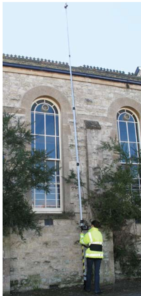
Figure 11 Remote inspection mast with hand-held lightweight CCTV system (Image courtesy of Survey Support Ltd)
