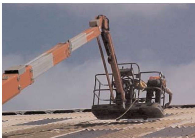
Figure 16 A mobile elevating work platform being used to replace a roof sheet
