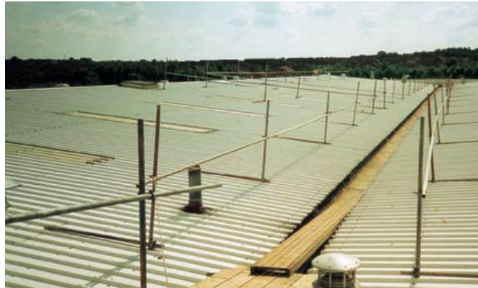
Figure 21 Demarcation barriers on a large, non-fragile roof, preventing access to the adjacent fragile roof lights. The roof lights are at least 2 m from the barrier
