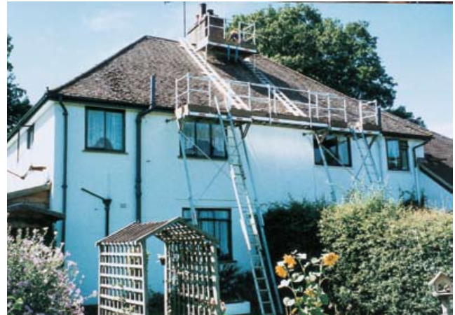
Figure 28 Proprietary system for access to roof and chimney
