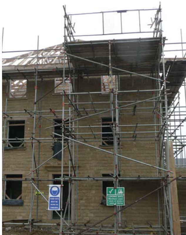
Figure 35 Scaffold loading bays can help to reduce material movement on the roof. Suitable barriers or gates should be provided to prevent falls at the open edge when loading is not taking place (Image courtesy of David Wilson Homes)
