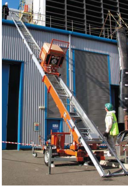
Figure 5(a) Industrial hoist (Images courtesy of HSS)
