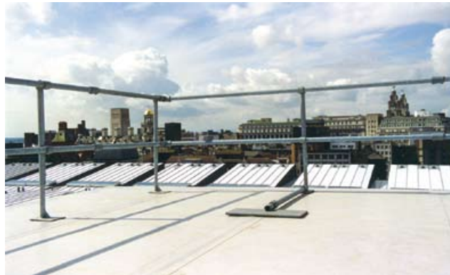
Figure 18 Temporary flat-roof edge protection. Adjustable supports enable work to progress with protection in place (Image courtesy of Safesite)
