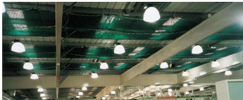
Figure 31 Safety netting used to provide protection for roof lights during minor roof works
