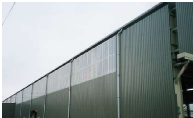
Figure 43 Lighting panels installed in the wall rather than the roof
