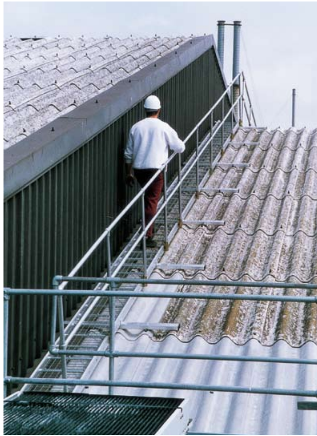
Figure 42 Permanent walkway giving safe access on a fragile roof. (This walkway was retrofitted, but similar access can be included in initial designs)
