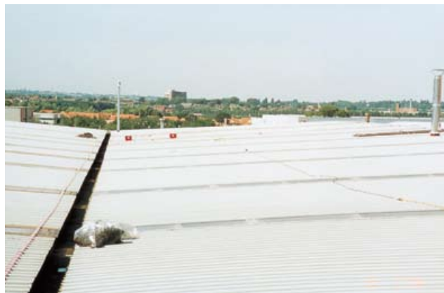
Figure 30 In some light conditions, it is difficult to distinguish the roof lights from the metal sheets on this type of roof. The valley gutter is very narrow and roof lights extend down to gutter level – both of these features increase the risk during cleaning, maintenance or refurbishment
