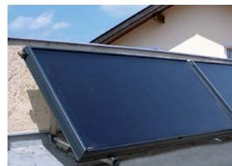
tecSol-Q installed on wall
