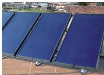
tecSol installed on rack
